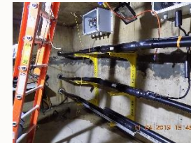
38 KV Power Line connects switch yard to substation.
